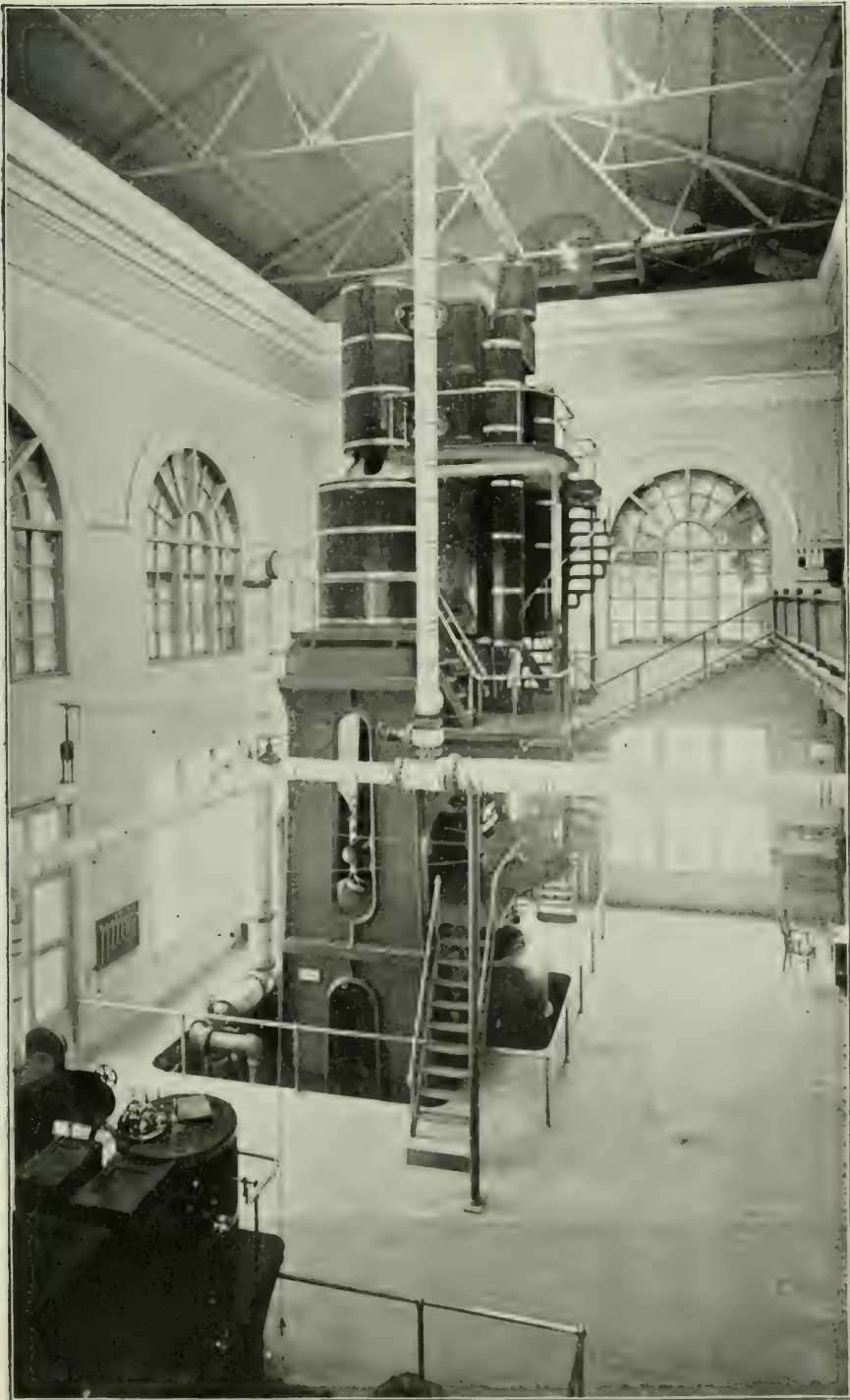
INTERIOR VIEW OF A PORTION OF THE PUMPING STATION.
